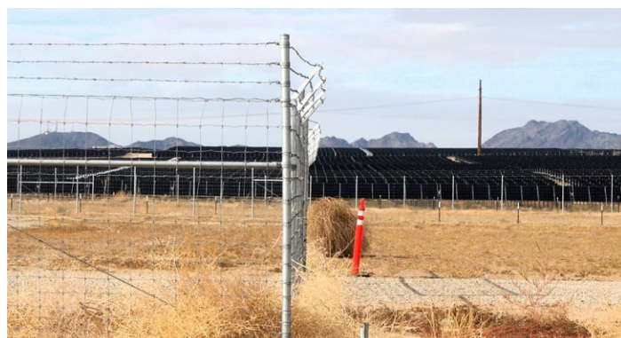
Solar farm enclosure in the southeastern California desert. Photo courtesy of the authors.
