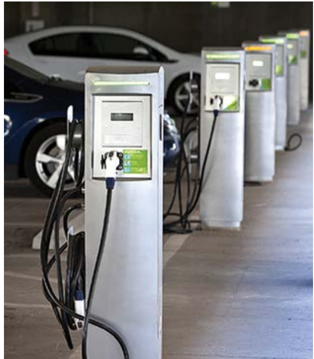
Electric Vehicle Charging. Photo credit: Dennis Schroder, National Renewable Energy Laboratory
