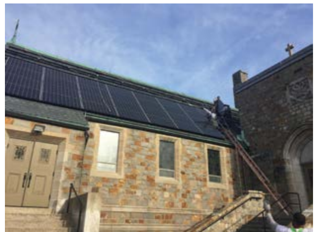
Solar Installation on Bethel AME Church in Jamaica Plain. Photo credit: Resonant Energy
