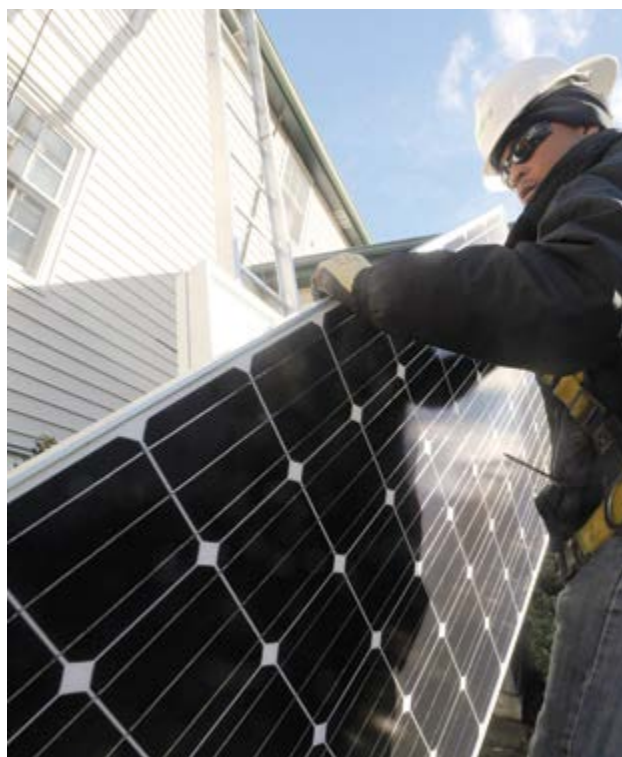
Solar roofs can leverage unused building space to generate renewable electricity. Photo credit: City of Boston
