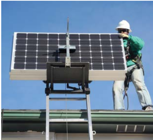
Rooftop photovoltaic installation. Photo credit: City of Boston
