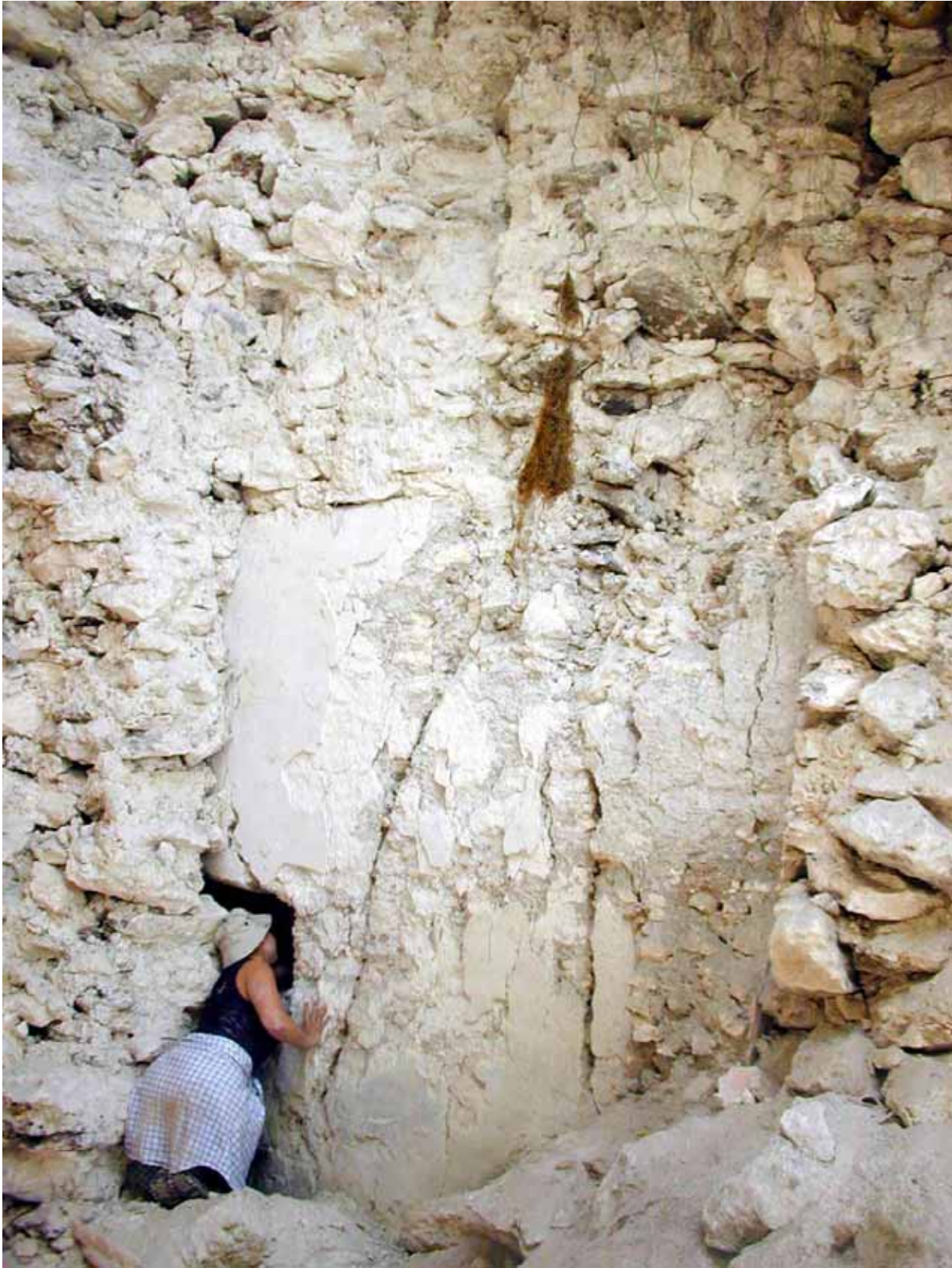
Figure 21. Interior of looters' trench in back of Cival Str. 1 exposing southern exterior wall and window in stucco-ed sub-structure.
