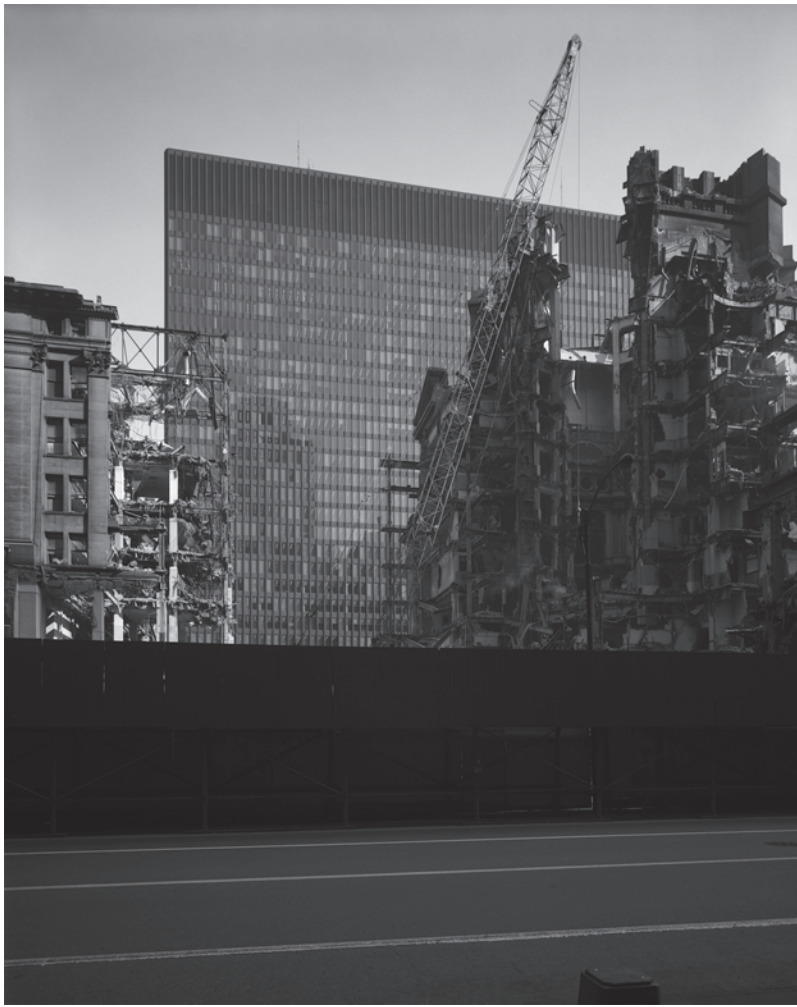
Figure 14 Henry Ives Cobb, Chicago Federal Building, 1896–1905, seen during demolition, 1965; in the background is Ludwig Mies van der Rohe’s Dirksen Courthouse in the Chicago Federal Center (HB-27043-M2, Hedrich-Blessing Collection, Chicago History Museum; © Chicago Historical Society, published on or before 2016, all rights reserved).
