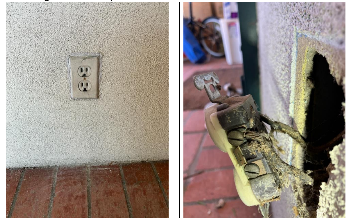
Figure 5. Outdoor patio outlet with 2-wire “end of circuit” termination
