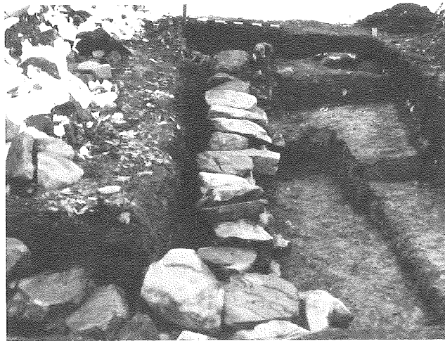
View of the foundation wall of the original East Ell during excavation.
