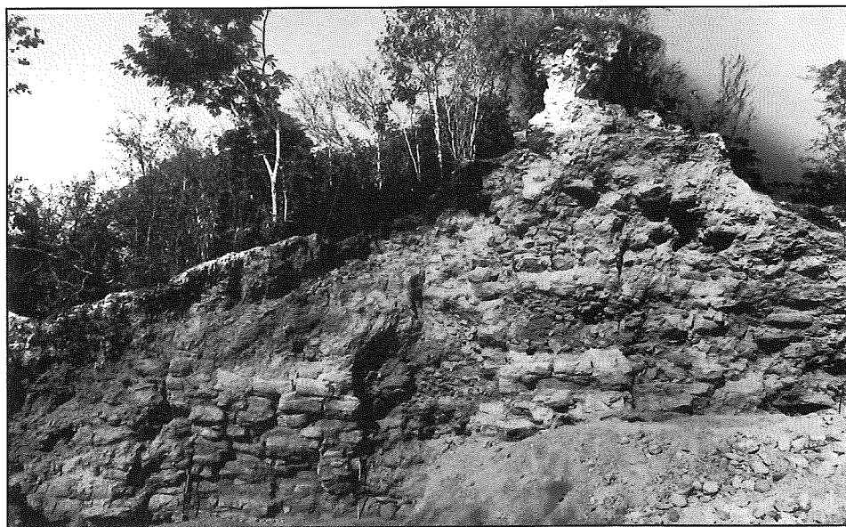
Structure 18 at Louisville, partly demolished for road fill in January 2000. Sections of limestone construction fill, laid side-by-side in "tasks" carried out by separate gangs of workers working simultaneously, have been exposed. Further destruction took place later in 2000; the site's other major pyramid was totally destroyed in 1999.
